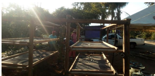
Figure 4 Shows the structure of how the prototype was built at Rancho Las Palmas
