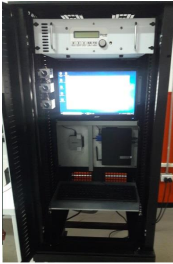
Figure 5 Cabinet with power source Source: Prepared by the authors
