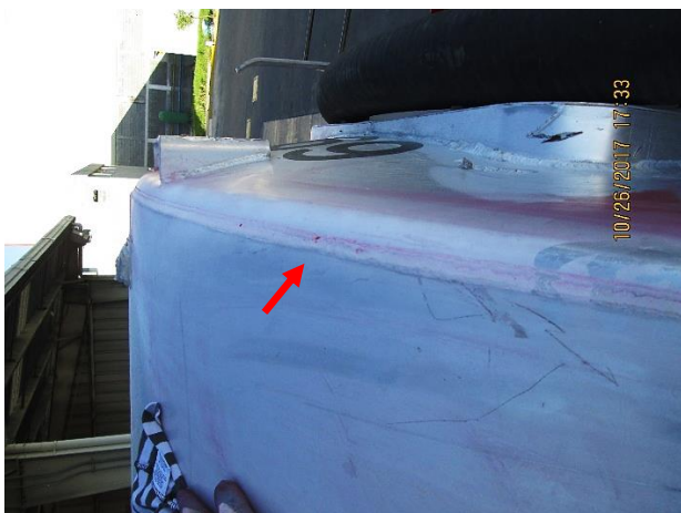
Figure 6 The image shows the results of the inspection by penetrating liquids in a previous repair by welding of the failed hopper. No indications were observed Source: own work [Canon powershot A3400IS]
