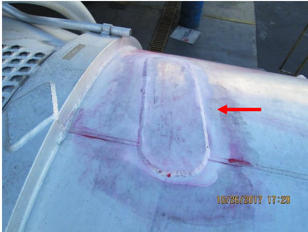
Figure 5 The image shows the results of the inspection by penetrating liquids in a previous repair by welding of the failed vessel. No indications are observed Source: own work [Canon powershot A3400IS]
