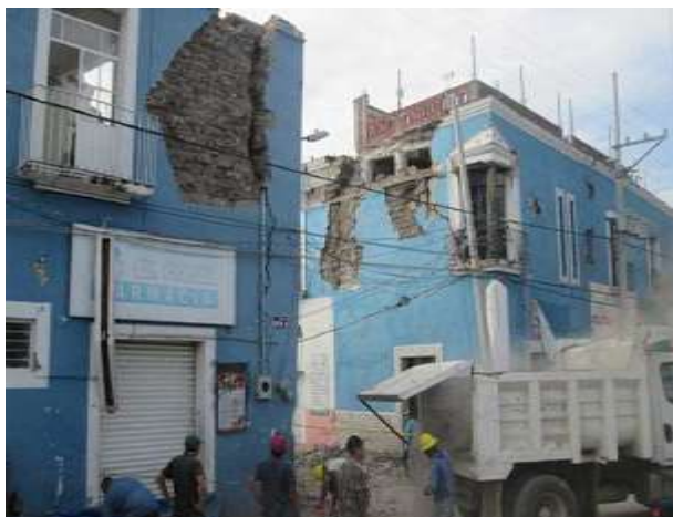
Figure 12 Unconfined walls, observed at the top of the wall, the separation of the wall with the roof Source: Cano, 2020
