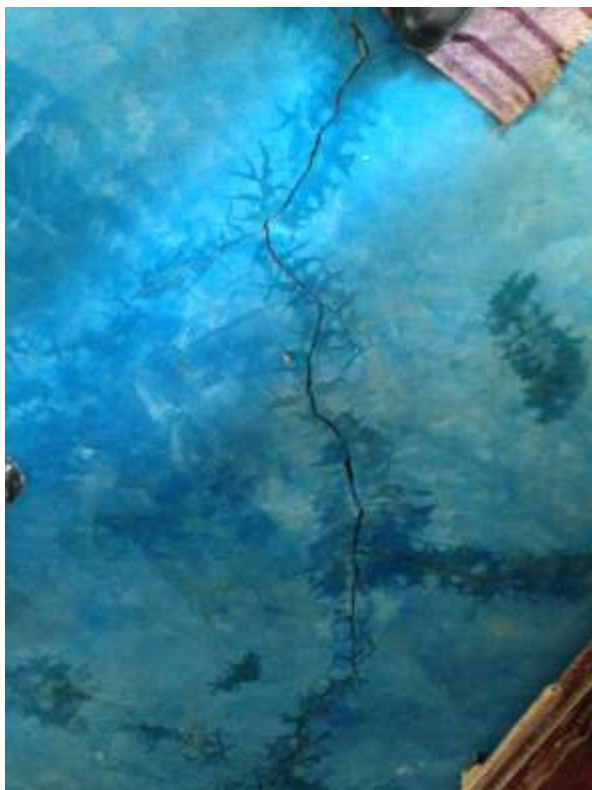
Figure 17 It was observed that there were already cracks produced by other earthquakes, in which the humidity caused more fissures than in the earthquake of 2017 were evidenced
