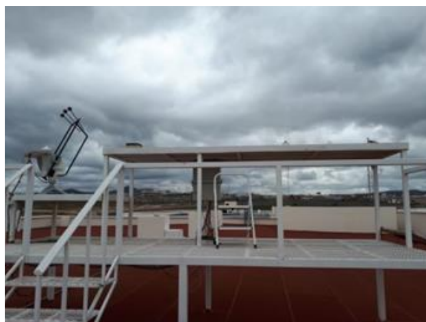
Figure 7 Solarimetric station Zacatecas_04
